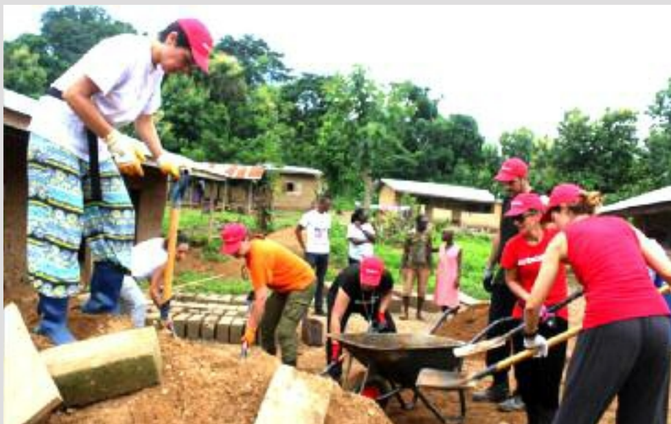
Child sponsors and volunteers from Greece contributing to the construction of teacher's quarters in Koru in the Kadjebi District of the Volta region
